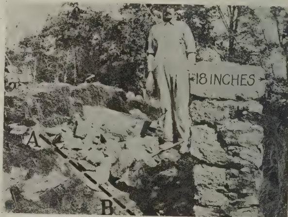
Fig. 2. Unsatisfactory cellar wall
